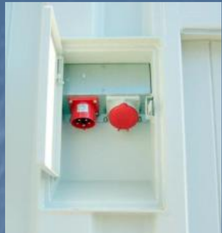
External Power hookup
