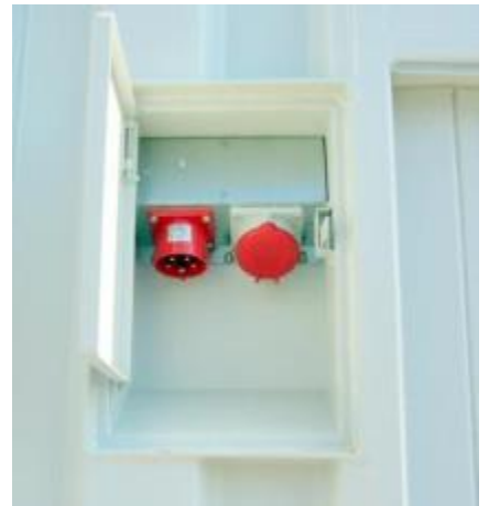
External Power hookup
