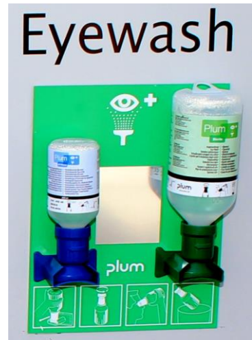
Emergency eye wash
