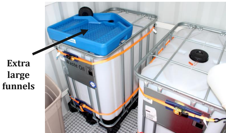
211 Gal or 800 l storage tanks for used oil & anti-freeze
