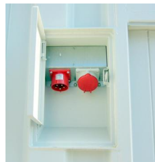
External Power hookup
