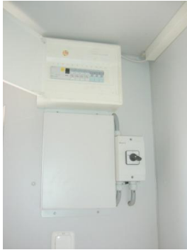
Main Power control Panel
